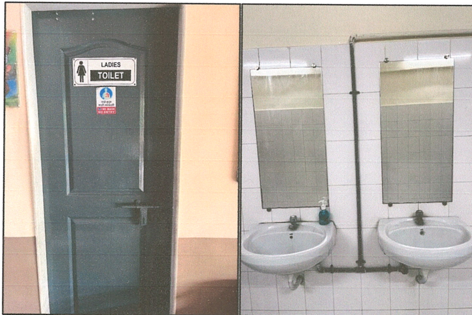
Ladies Washroom equipped with proper locks, mirrors and washbasins
