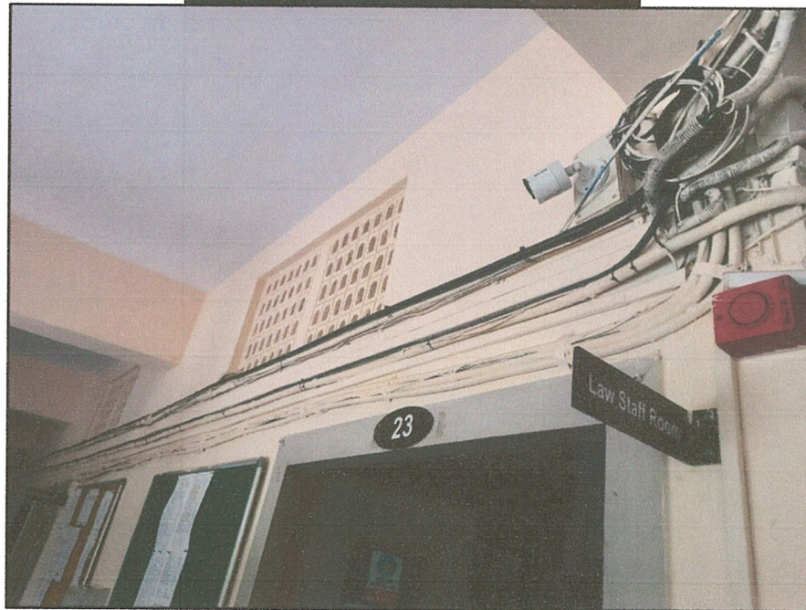
CCTV surveillance in the college building
